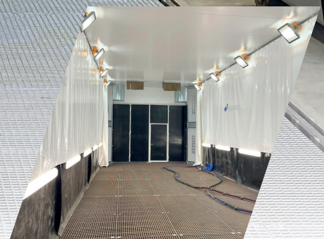
COMBINED BLASTING AND PAINTING (ALL-IN-ONE MULTI-PURPOSE CHAMBERS)
